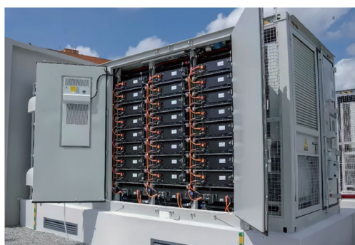
(a)液冷式储能电站
